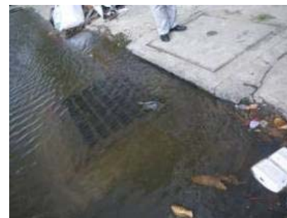
Canal water flows backward through street inlet
