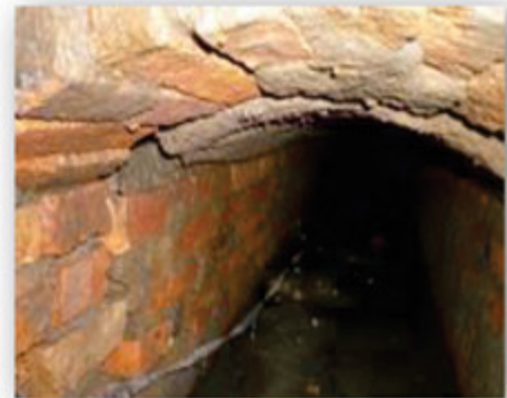
老朽化が進んだ下水管 Sewer pipe with aging
