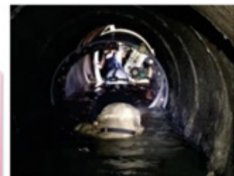
管路更生工法の施工状況 Pilot construction of Pipe Rehabilitation Technology (September 2015)
